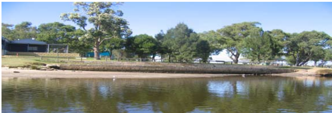
Figure 7.2 Overtopping, lack of drainage management, absence of filter cloth and re-grouting – Qantas Boat Ramp
