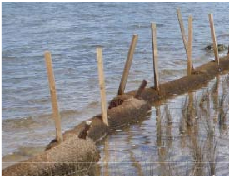
Figure 3.3 Stakes too long and pushed through centre of log instead of either side
