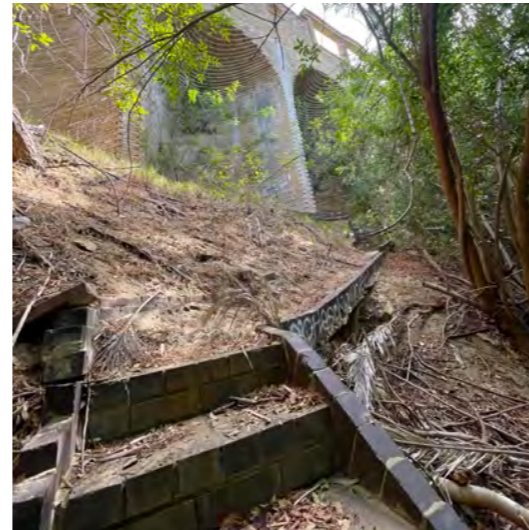
Fig: Brick stair and walkway undermined
