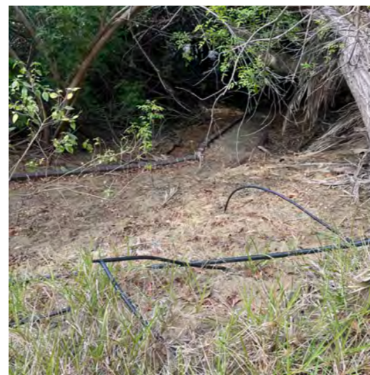
Fig: Remnants of irrigation, weeds and grasses
