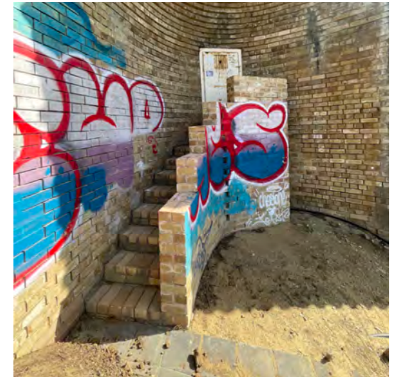
Fig: Staircase entrance to site, graffitied
