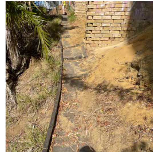
Fig: Undermined walkway and yellow sandy fill
