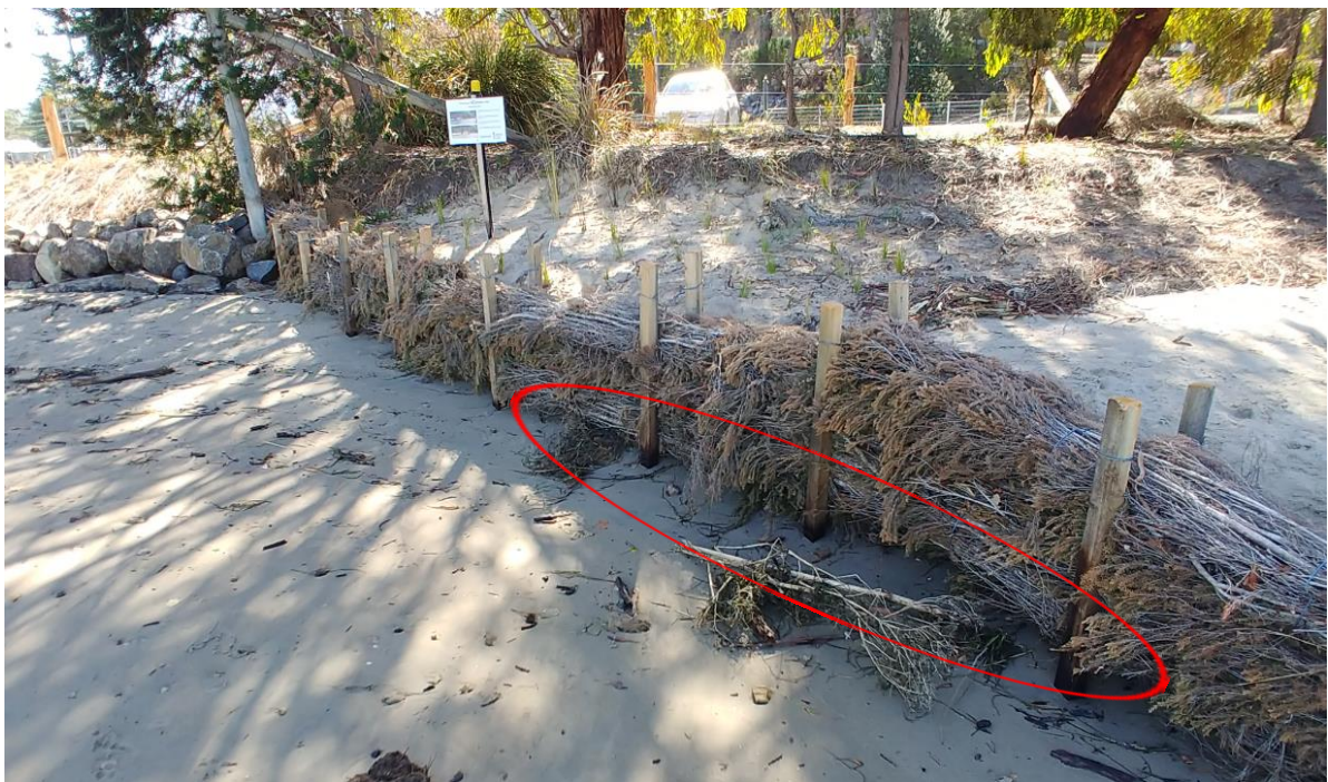
Figure 9 Use of brushwall without toe protection causing undercutting and erosion (Source: Syrinx)
