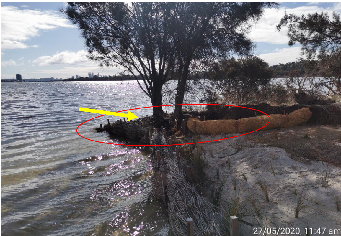
Figure 6. Example of a low height brushwall causing overtopping and bank erosion (Source: Syrinx)
