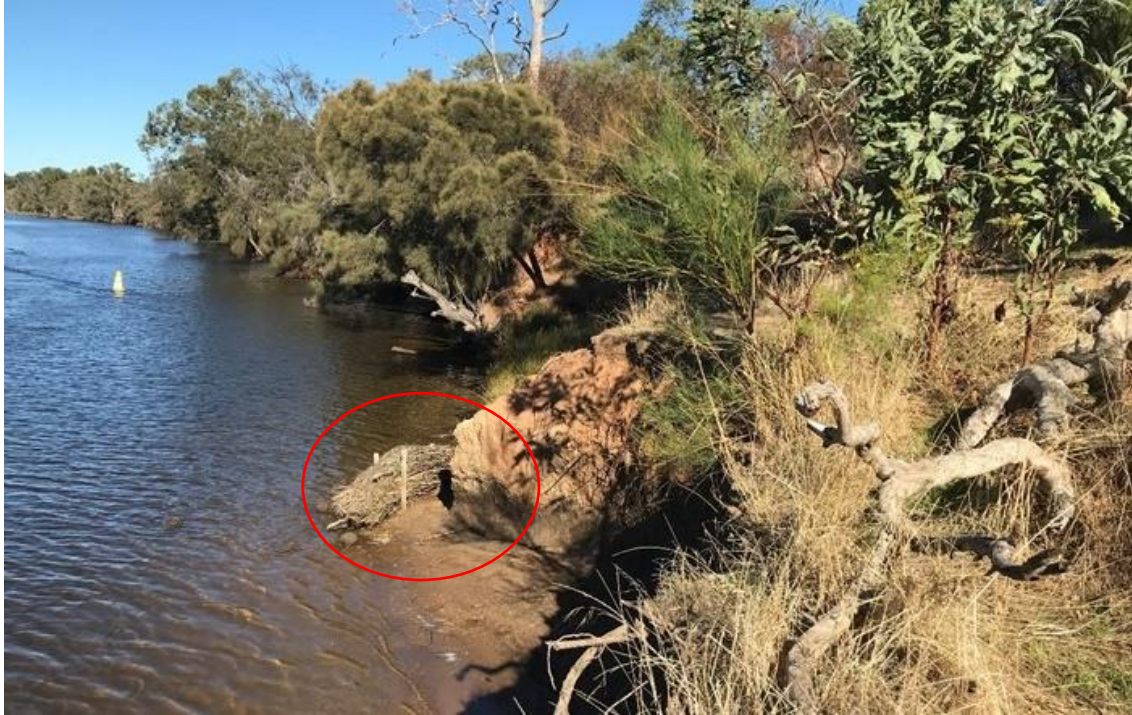
Figure 7 Incorrect tie in with the bank (Source: Syrinx)
