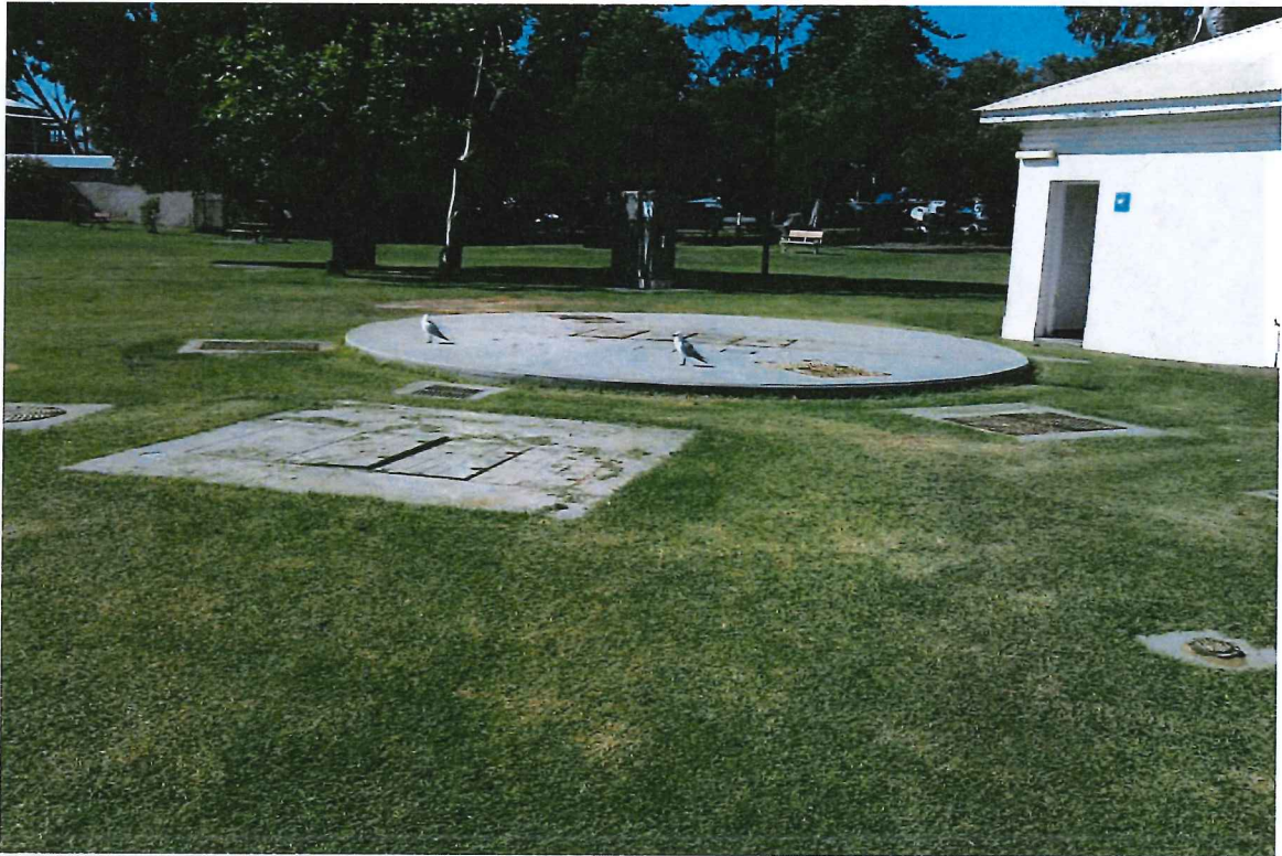
3. Sewer mains pump station and overflow tank with inspection manholes to be retained
