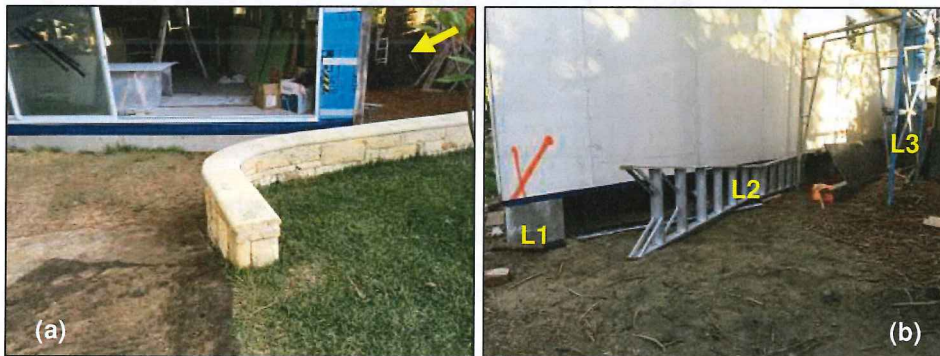
Figure 6. (a) & (b) Construction of a new workshop within several metres of a mature 30m+ tree (see arrow) using three lintels (L1-3) attached to screw pile footings and spanning across the rootplate of the tree, alleviating damage to the large woody roots responsible for tree stability and maintaining aeration to the small non-woody roots within the upper soil profile and located further away from the trunk N.B. the depth of each lintel in contact with the ground surface is less than 100mm (hand digging used) and each lintel is connected to approximately eight screw piles.
