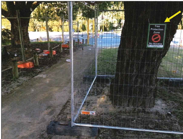
Figure 2. Protective fencing comprised of 1.8m high chain-wire mesh panels and signage providing information (see arrow) regarding access within the fencing should be erected prior to the commencement of construction activities that involve machinery and have the potential for collision injury.
