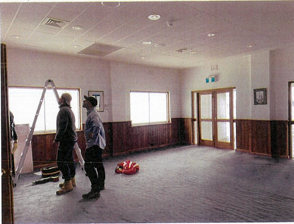
Photograph 09: View of the northeast wall, which is to be modified, to allow access to the new lift and UAT area. Griffiths Architects, August 2022.
