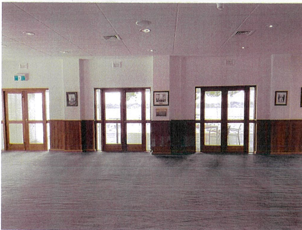
Photograph 08: View of the southeast wall, which is to be opened up and connected with the existing deck. Griffiths Architects, August 2022.
