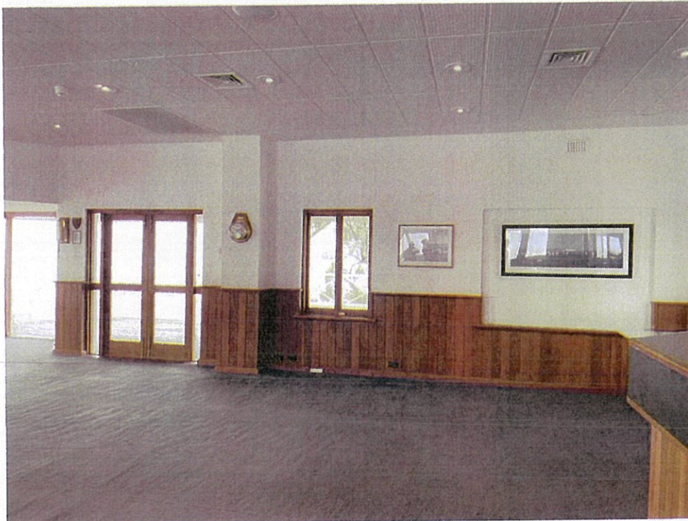
Photograph 06: View of the southwest wall, which is to be opened up and connected with the existing deck. Griffiths Architects, August 2022.
