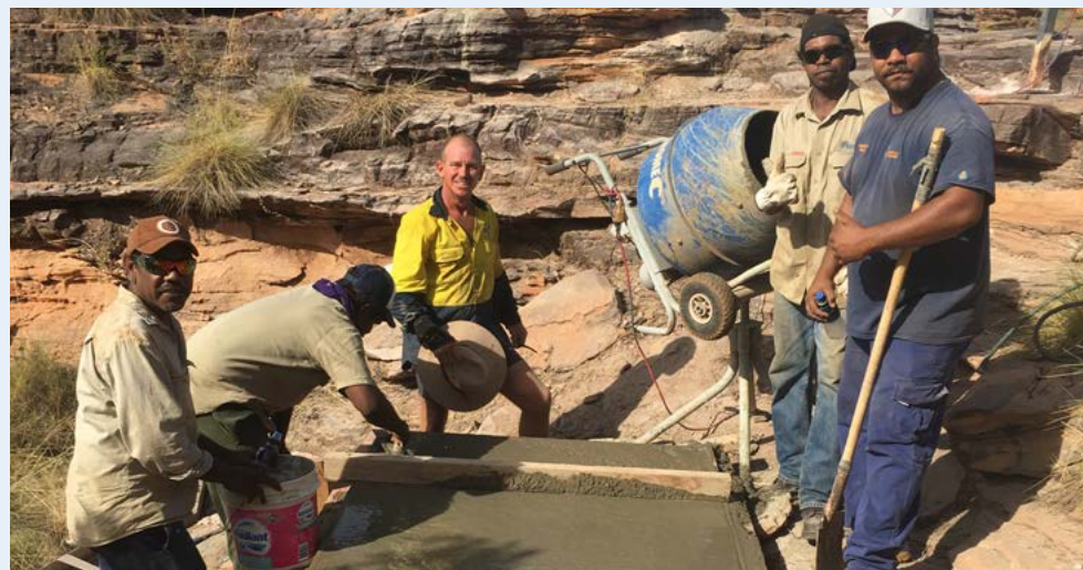
MG rangers installing a new staircase in Mirima National Park. Photo – DBCA
