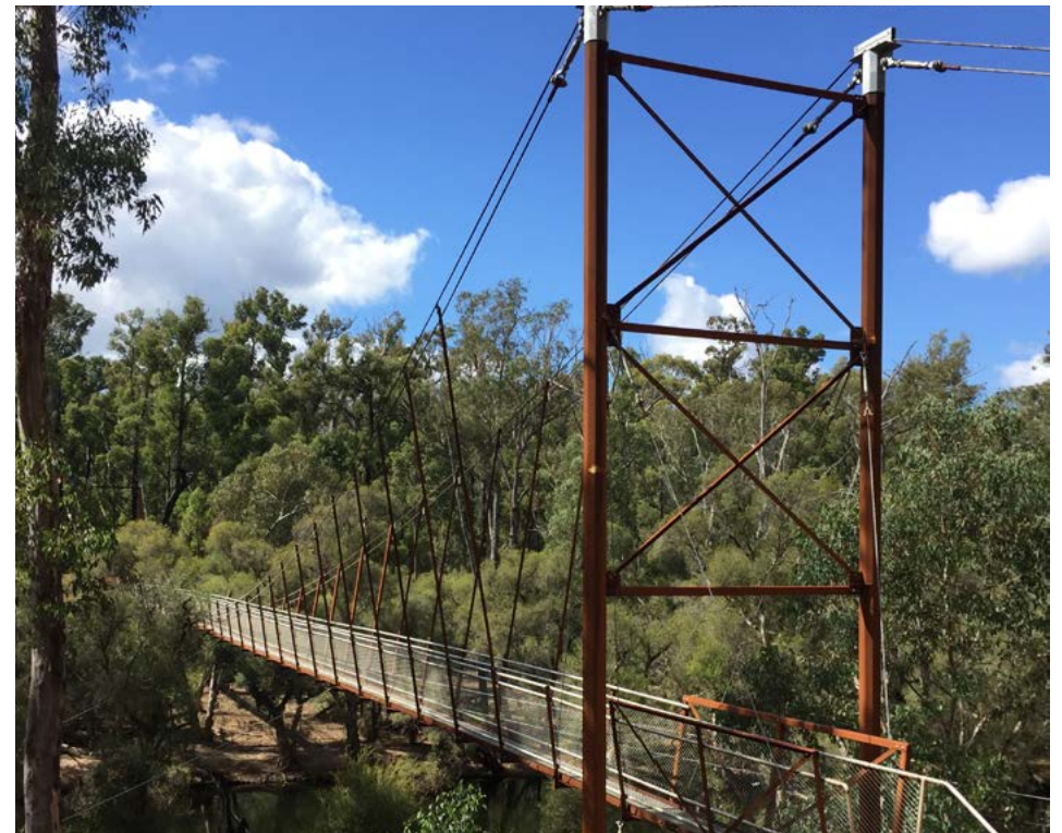
The new Bilya Bjena Bidi suspension bridge spans 82m across the Murray River in Lane Poole Reserve. Photo – Stuart Harrison/DBCA
