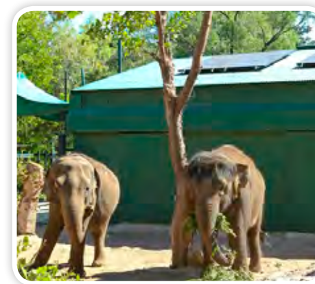
Solar panels on the elephant barn
