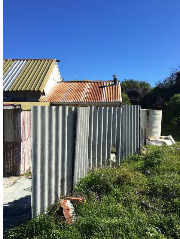
Photo 5. Suspect ACM fence adjacent to Wedge shack W245, where AF sampling was conducted.
