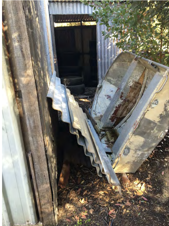
Photo 20. Typical occurrence of suspect ACM sheets (G85).
