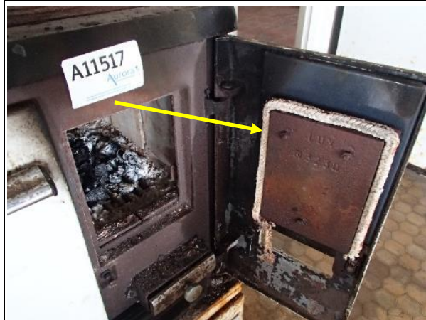
Chrysotile rope seal to oven door. Shack G120
