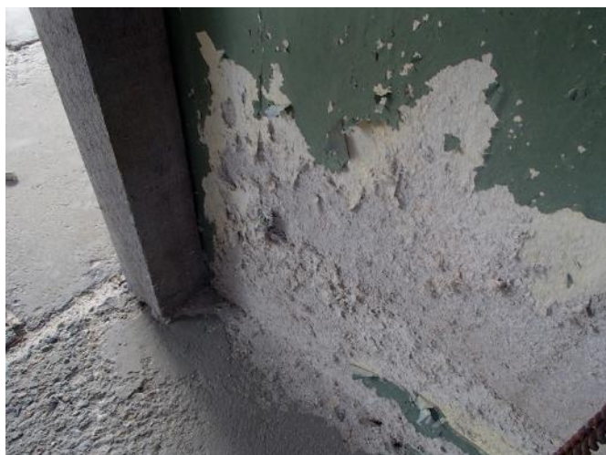
PHOTO: Heavily weathered asbestos cement external wall cladding to shack W253.
