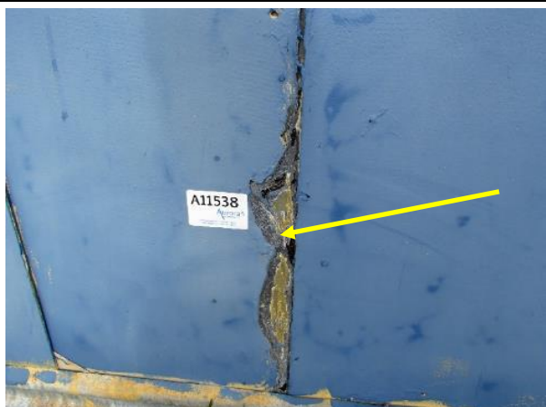
Bitumen adhesive under external wall panels. Shack W313
