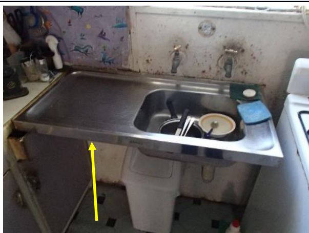
Bitumen sound dampener membrane to underside of sink. Shack W76.
