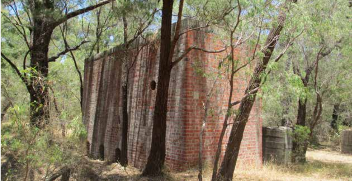
Brick drying kiln at the former Lake Clifton lime works site in Yalgorup National Park. Photo – Grace Patorniti/ Parks and Wildlife
