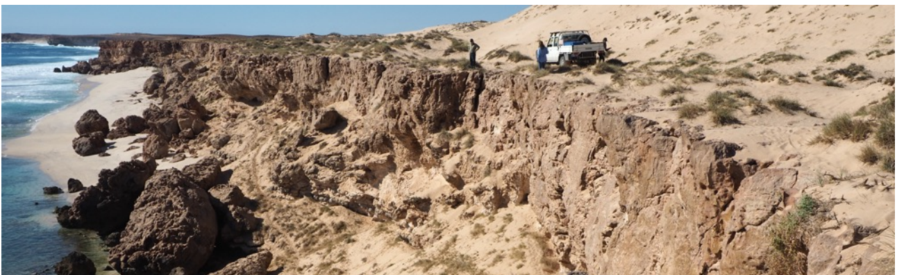
This vehicle track close to cliff edge, south of Tombstones has been closed due to visitor risk. Photo - Emma West/DBCA
