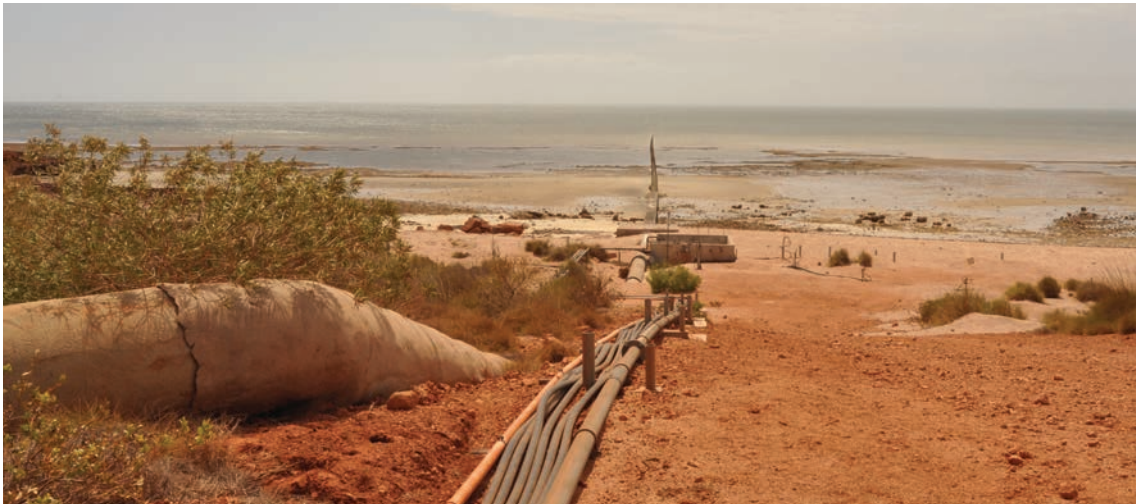
A significant amount of infrastructure exists on Barrow Island Nature Reserve including this tanker loading pipeline on the east coast, near Town Point. Photo – Kevin Crane
